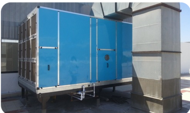
AIR WASHER UNIT WITH DUCTING
