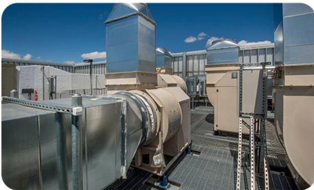
SUCTION UNIT WITH DUCTING
